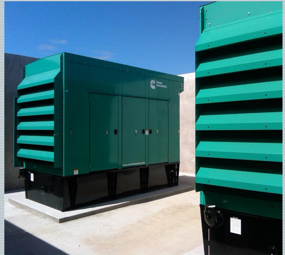
Future Redundant Generators
